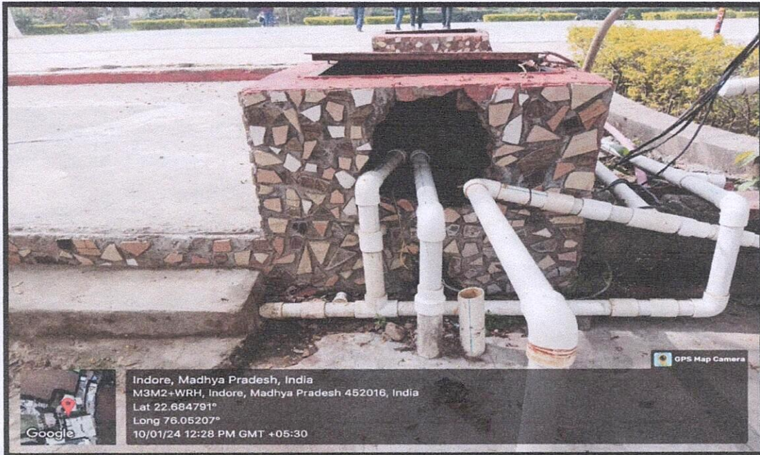
Water distribution pipes -Underground Water Tank
